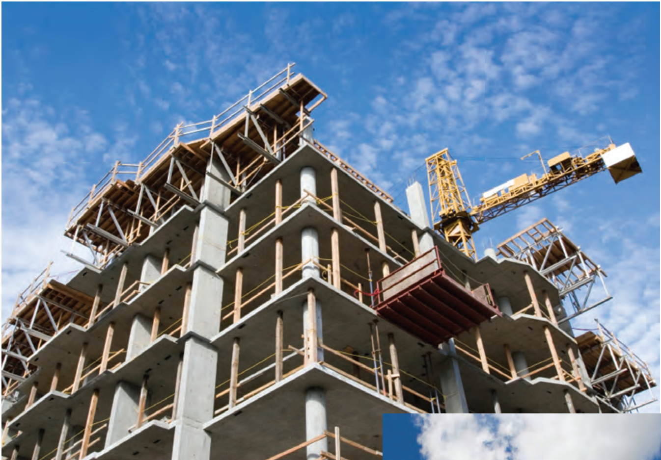
Construction Elevator Emergency Stops
