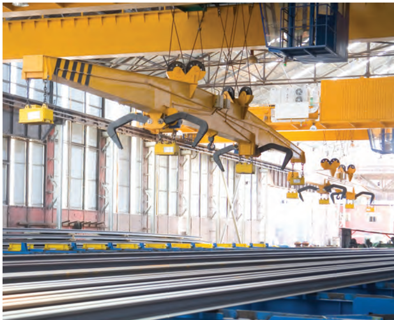
Material Transport Crane Applications
