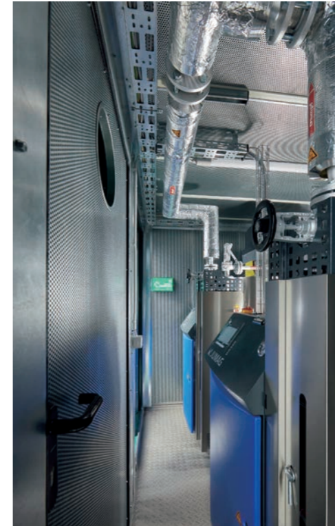
Fig.: Inside, Steam system
