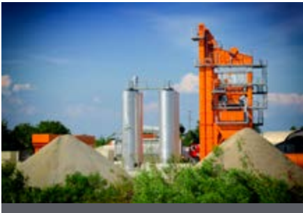
Asphalt mixing plants
