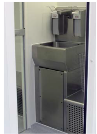
Personnel air lock area with washstand
