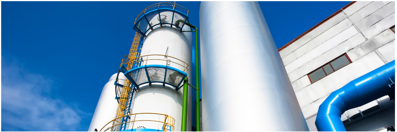
Air Separation Plant
