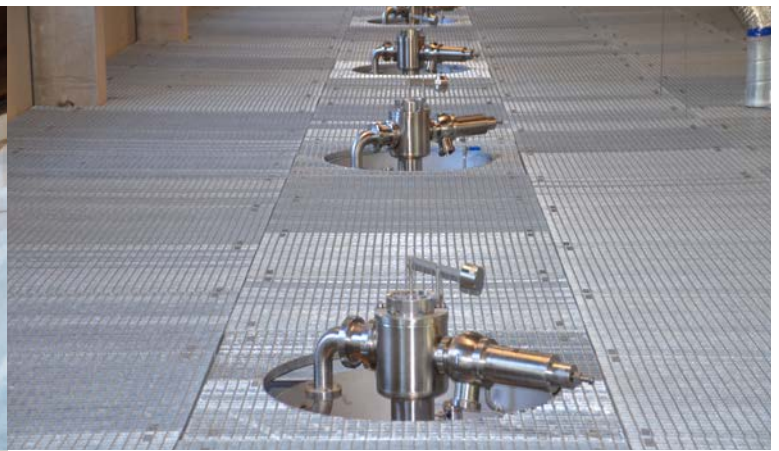
↶ Safety valve on a bioreactor
